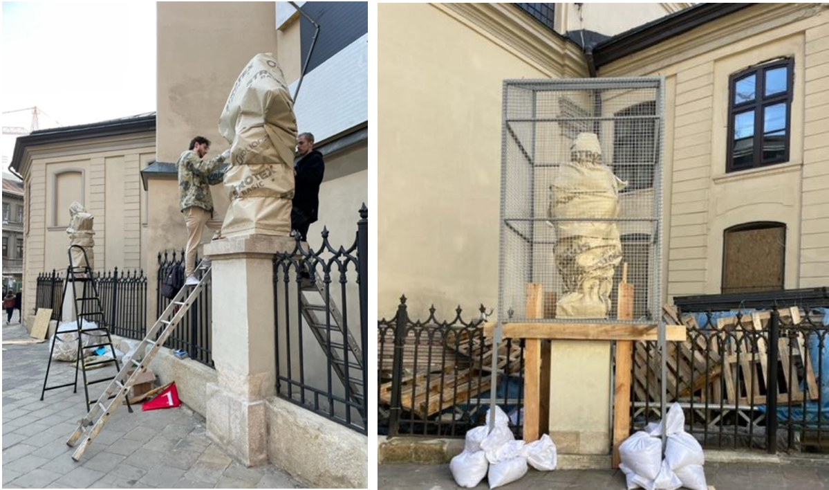
Figure 3. Preventive action to protect the cultural monuments in the city of Lviv, Ukraine
